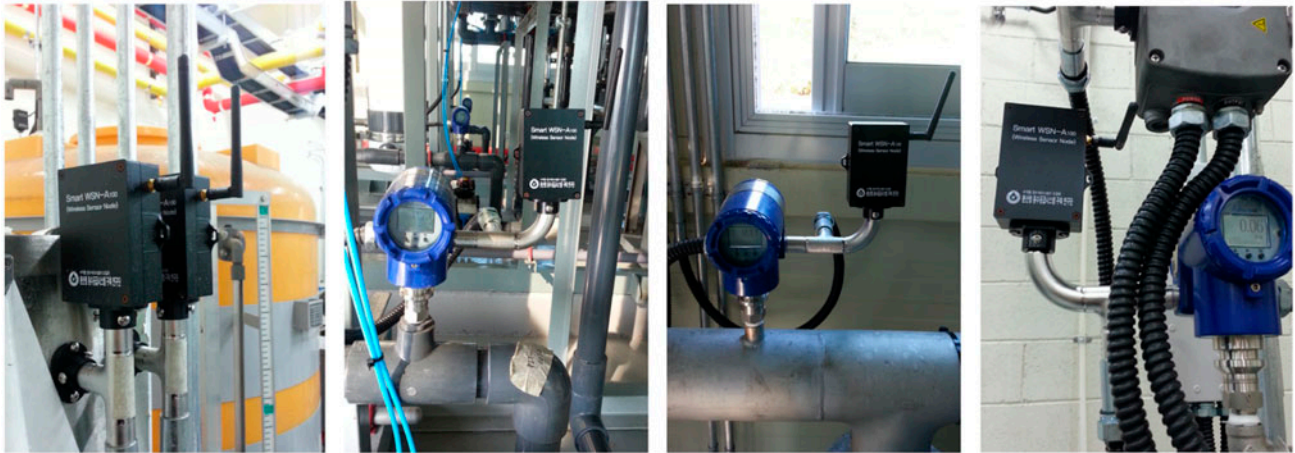
Fig. 4. Installed sensor nodes.
