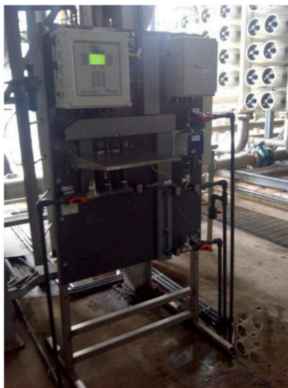
Fig. 1. 3DT for membrane skid installed at site.
