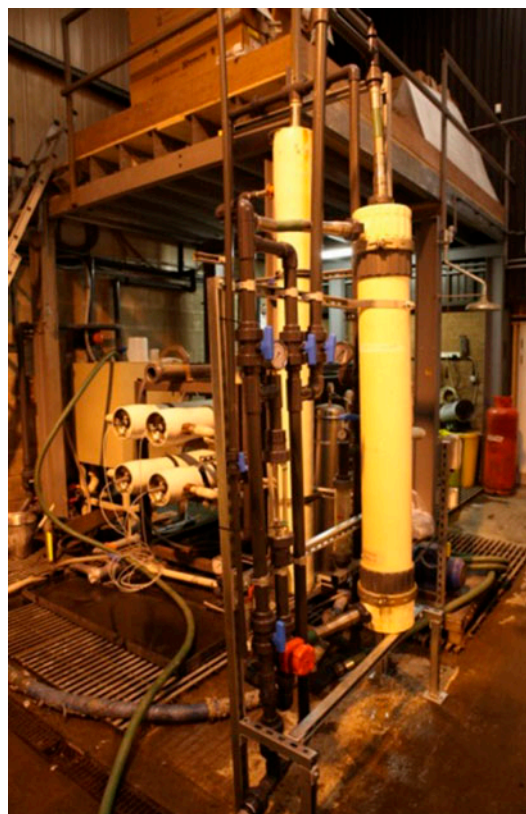
Dow UF module under test, with Pall module in background
