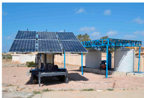
Fig. 7. Mobile PV/RO water desalination plant.
