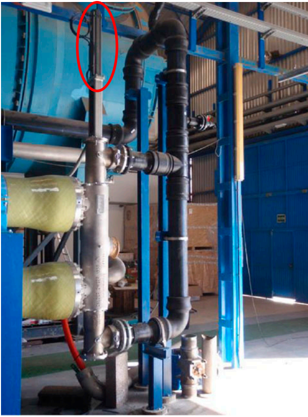
Fig. 9. Desalination plant of Morrojable with electric actuator and FRP vessels.
