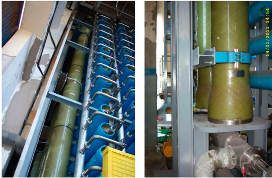
Fig. 6. Construction of the new membrane racks and equipment with the DWEER installation in vertical position. Note the Lynx™ control valve mounted underneath.
