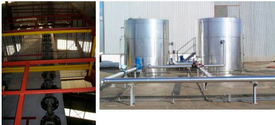
Fig. 14. View of the solar MED plant at PSA/CIEMAT and thermal storage tanks.
