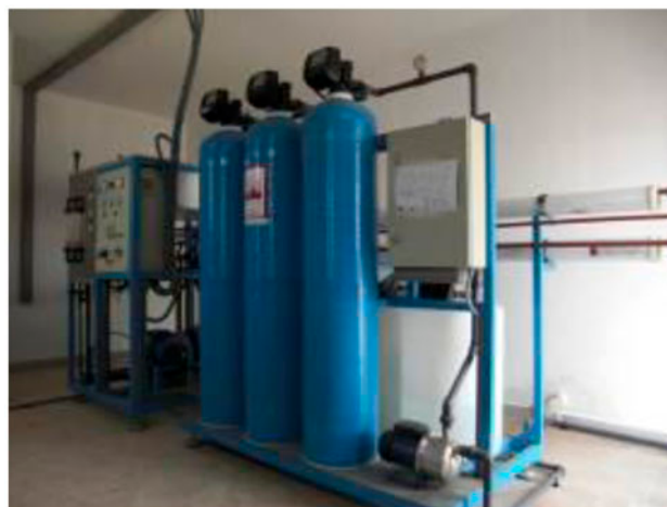
Fig. 9. View of a 1 m 3 /h RO unit installed in Morocco. Source: ITC.
