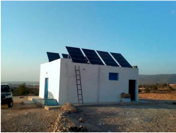
Fig. 10. The installed 4 kWp PV system, Morocco. Source: ITC.
