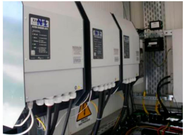
Fig. 5. View of the inverters, Strogili island, Greece.
