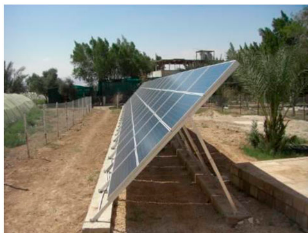
Fig. 8. The installed 10.4 kWp PV system, Jordan Valley. Source: NERC.
