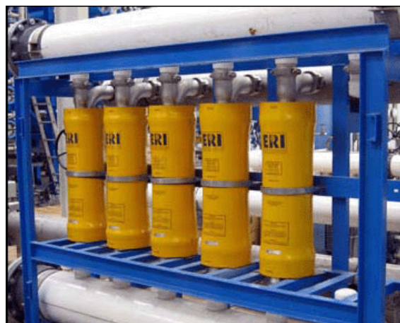
Fig. 1. PX-220 Energy Recovery device array.
