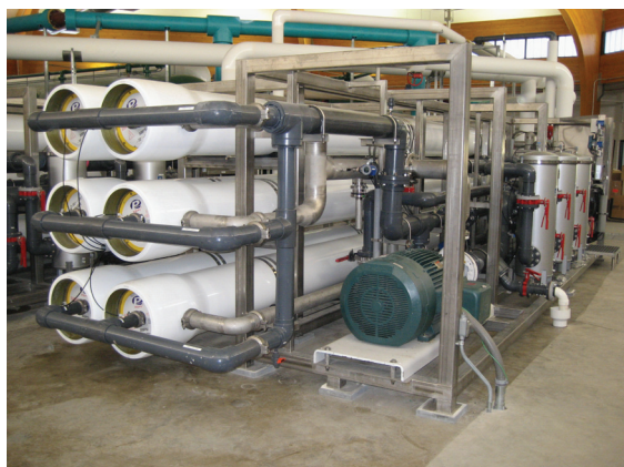
Fig. 3. City of Waupun RO train.
