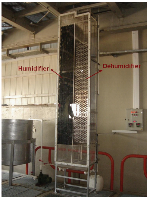
Fig. 3. Humidifier and dehumidifier towers of HD desalination unit.
