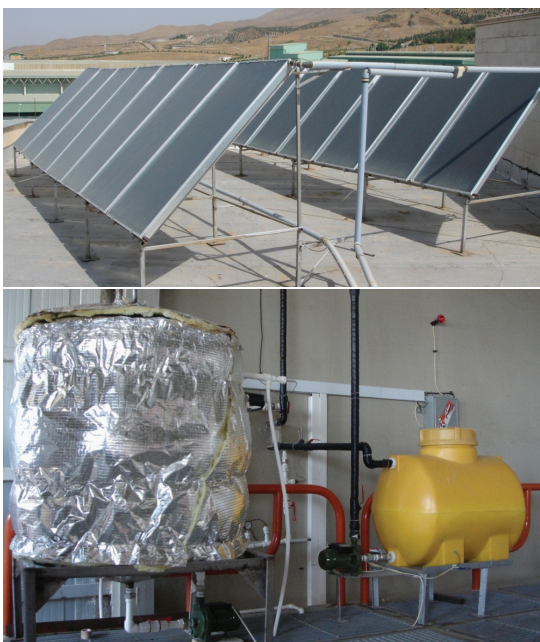
Fig. 4. Collectors and hot water storage tanks of HD desalination unit.
