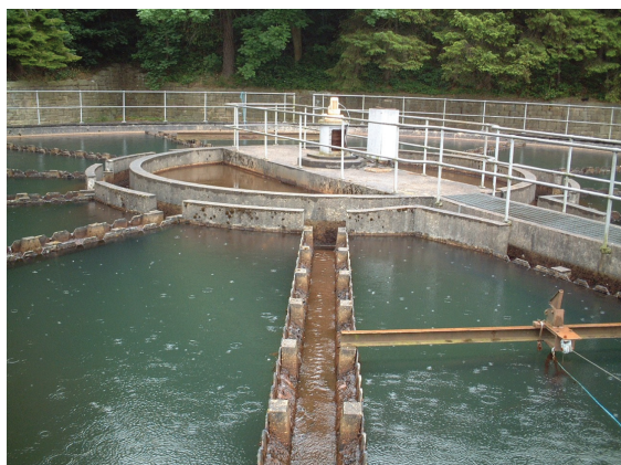
Fig. 1. Solids-contact unit for clarification (Courtesy: Severn Trent Water).
