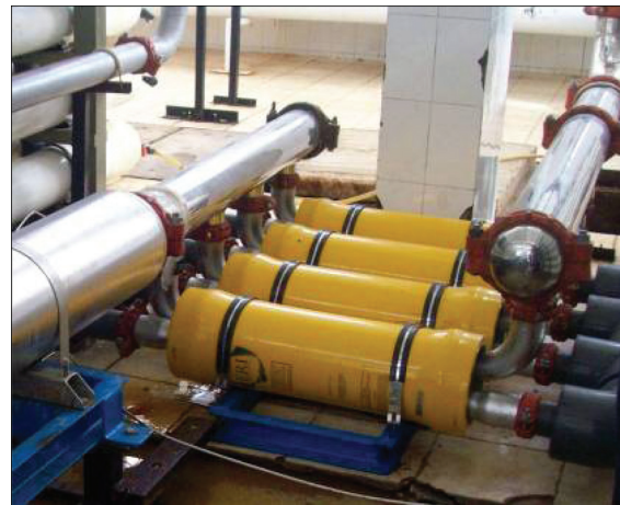
Fig. 8. PX device installation at the Sina plant.
