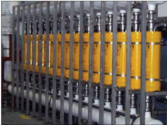
Fig. 6. PX installation in the Las Palmas III plant.
