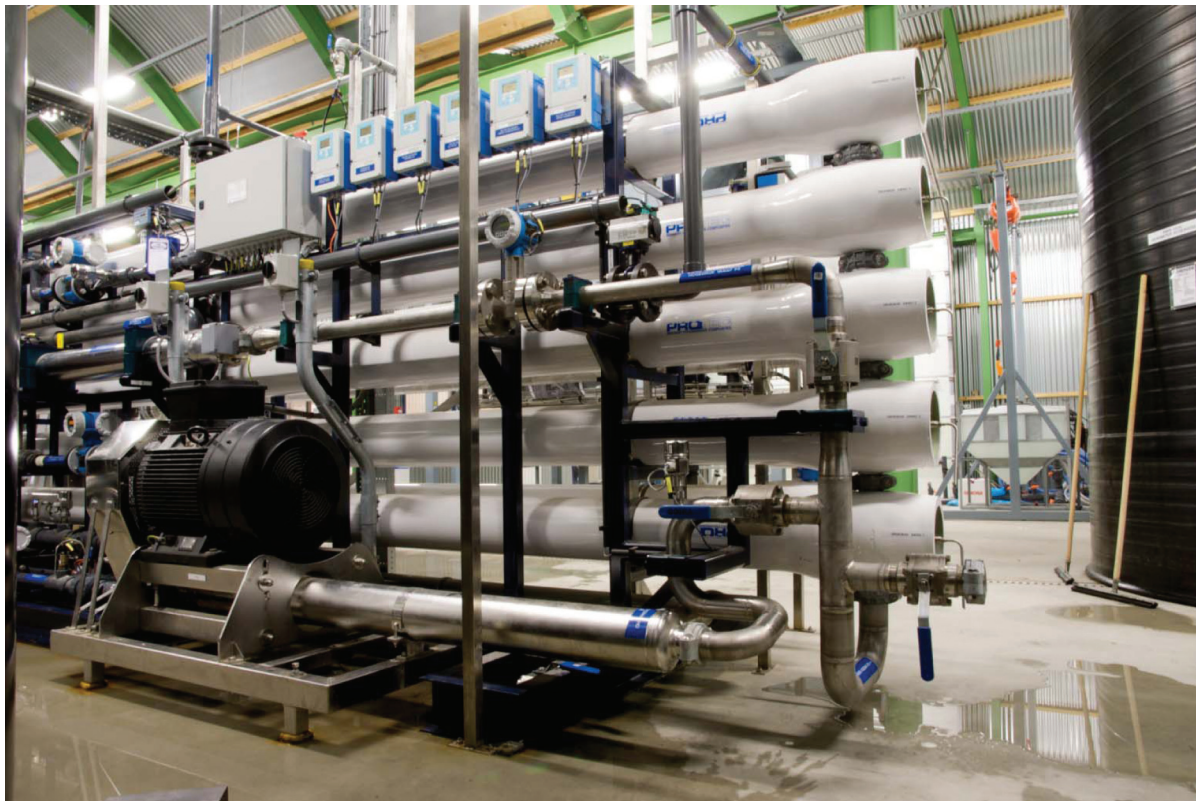
Fig. 4. Grundfos BMEX system on SWRO unit
