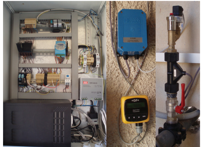
Fig. 8. Automation panel, instruments, sensors. Left: Automation panel contains: UPS, power supply, fusing, web i/o module, relays, surge arrestors and cabling. Middle: Instruments. Right: Sensors.
