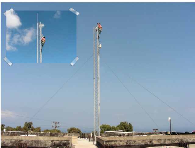
Fig. 5. Main antenna tower over water company.
