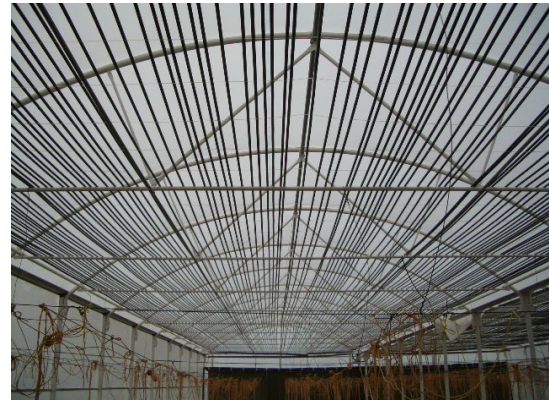
Fig. 3h. Solar heating pipes [8].
