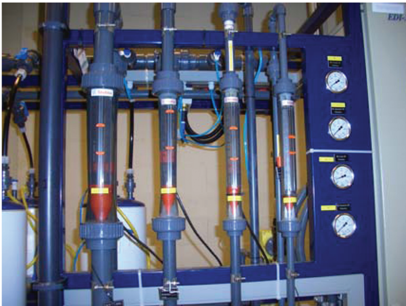
Fig. 6. Flowmeters and manometers used in the system.
