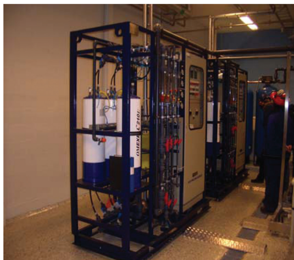
Fig. 5. Photo of the two DOW EDI skids used at Storuman power plant.
