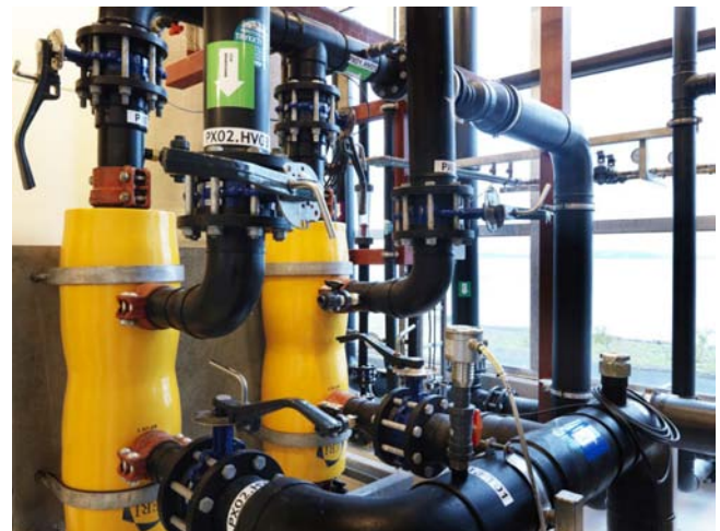
Fig. 6. 2 energy recovery devices recycling the PRO pressure.
