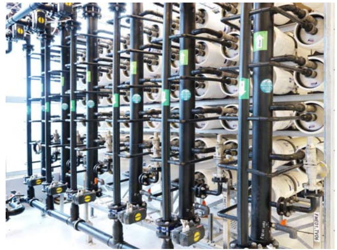
Fig. 5. The PRO membranes with pressure vessels and PE piping.
