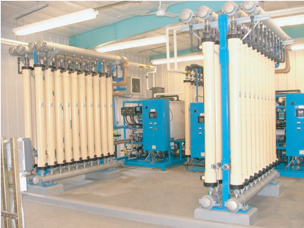
Fig. 3. Pall Microfiltration System.
