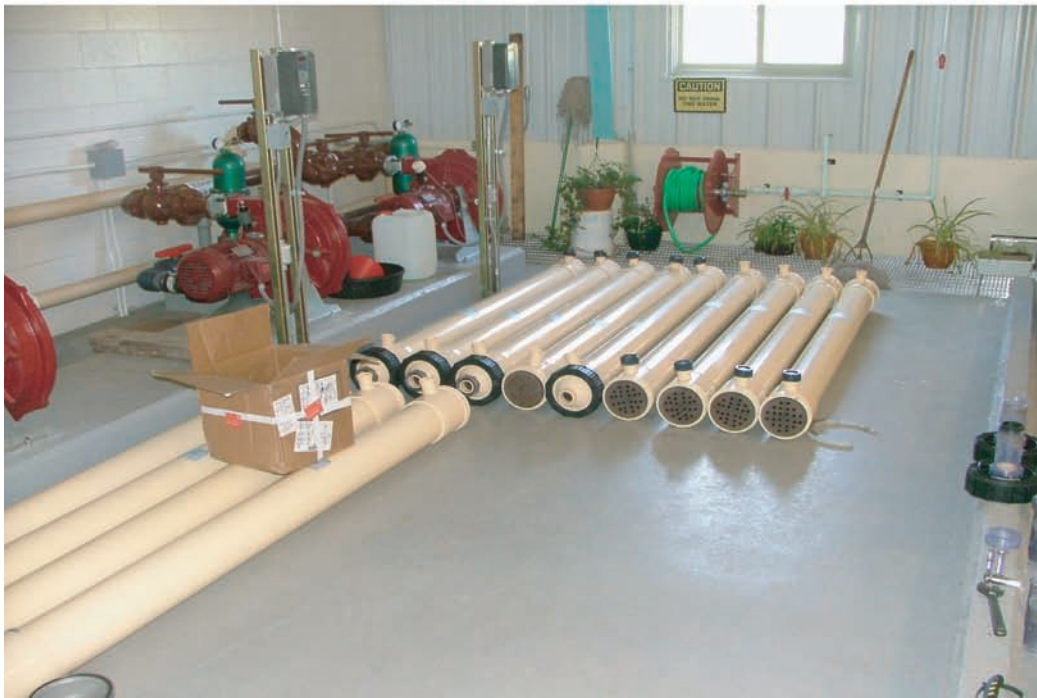
Fig. 4. Pall Microfiltration System – Rack A reconfiguration.
