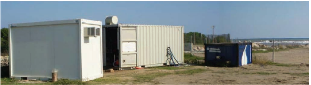
Fig. 1. Pilot plant, Neodren pumping station (right) and office container (left) beside the beach near Barcelona airport. Source: Ulbricht / MEMBRANA.
