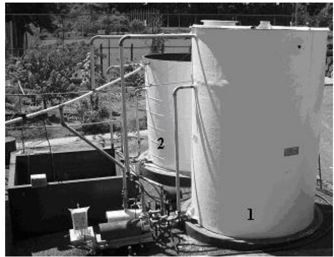
Fig. 2. Installation of the ASBBR (1) and the storage tank (2).
