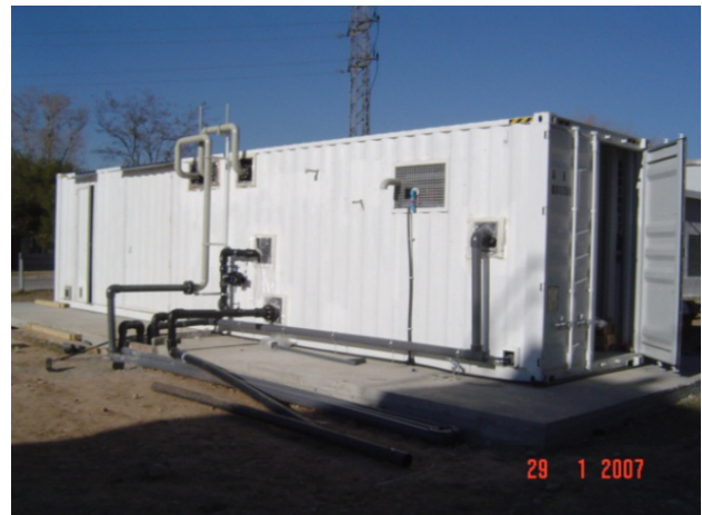
Fig. 2. EDR pilot plant at Abrera DWTP.
