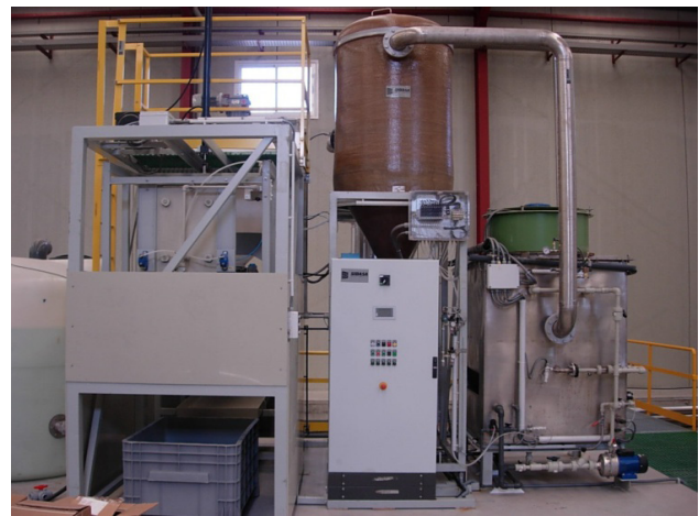
Fig. 5. Evaporation pilot plant II.
