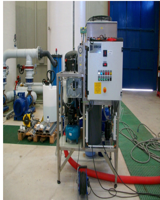
Fig. 4. Evaporation pilot plant I.
