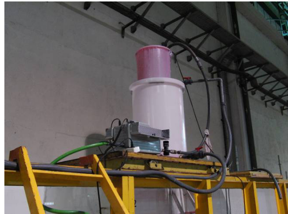
Fig. 14. System to prevent flow fluctuations due to variations in the water column over the pumps work.
