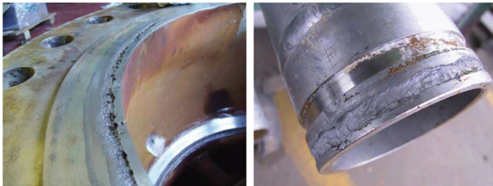
Fig. 16. (a) Crevice corrosion of a cast superduplex stainless steel at gasket location, (b) crevice corrosion of a wrought superduplex stainless steel at a “Victaulic-type” connection.
