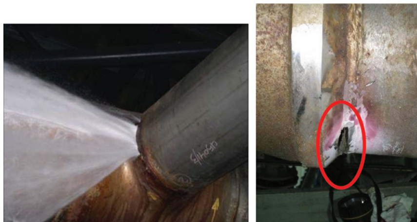
Fig. 17. Perforating pitting corrosion at welds on superduplex stainless steel pipes. In these cases, welding was not performed according good engineering practices.
