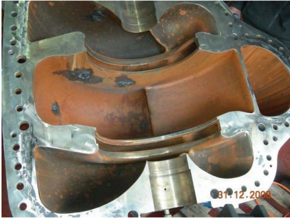
Fig. 14. Overview of the corroded pump made of cast super duplex stainless steel ASTM A890 Gr5A.
