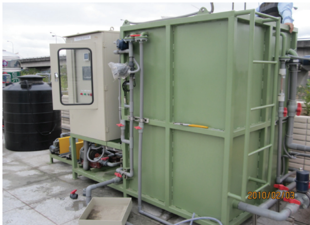
Fig. 5. Full-scale BioMF system for carwash wastewater reclamation.
