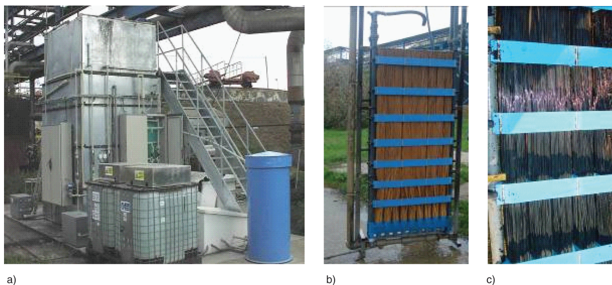
Fig. 3. Photo documentation: A - overview of pilot model unit, B - module after chemical regeneration, C - module before chemical regeneration.
