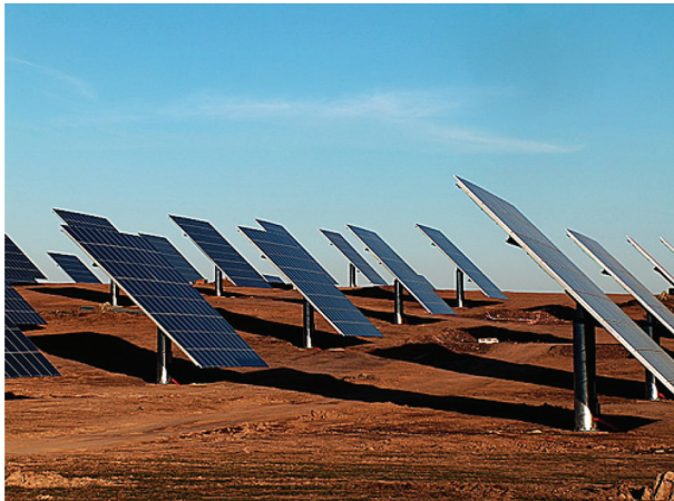
Fig. 8. Moura PV power plant in Portugal [15].
