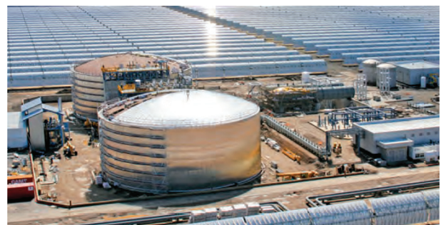
Fig. 11. Andasol solar power plant, parabolic trough power plant with molten salt thermal storage [19]
