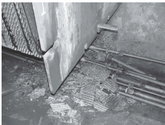
Fig. 1. Thermo-vapour compression unit during a cleaning section.
