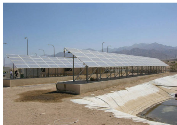
Fig. 3. 16 kWp PV plant, Aqaba, NERC, Jordan.
