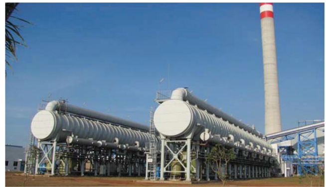
Fig. 5. The installation site of 2 \times 4,500 \text{ m}^3/\text{d} MED device: (a) hoisting of evaporator and (b) the panorama of desalination host after installation completely.
