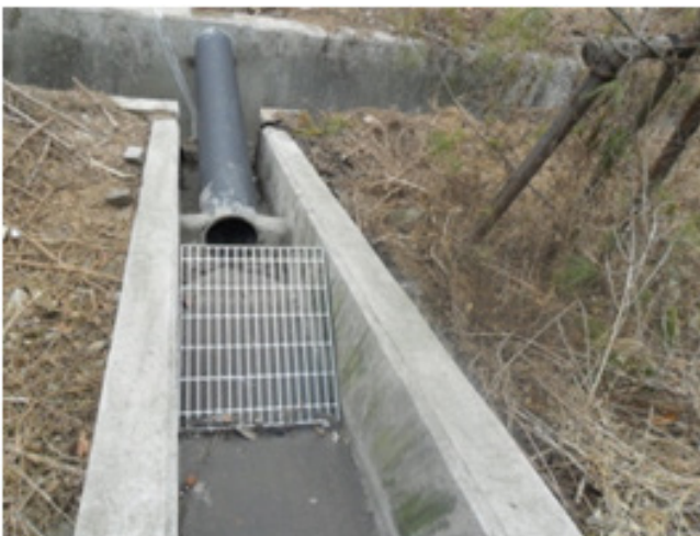
Fig. 5. Inflow screen installation error.
