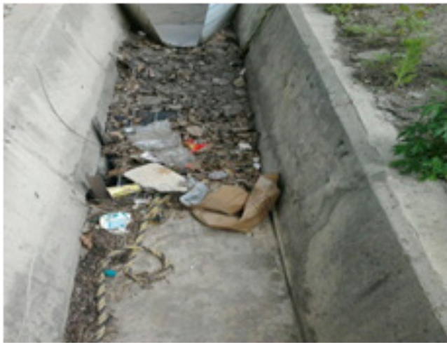
Fig. 3. Clogging of inflow screen.
