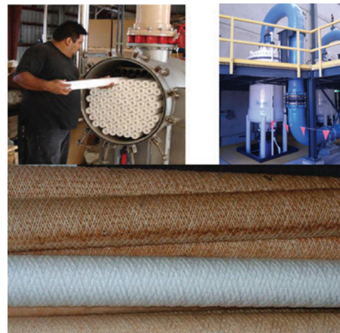
Fig. 6(c). A cartridge filter in a horizontal vessel (upper left) and a vertical vessel (upper right) with a differential pressure measurement (Perth) [13, 6].
