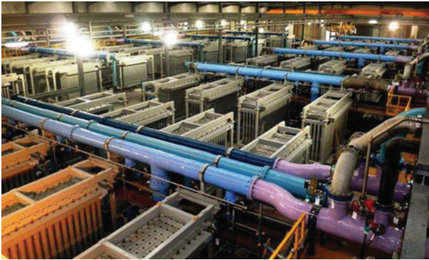
Fig. 22(a). Perth II – Memcor pressurized pretreatment system [13].
