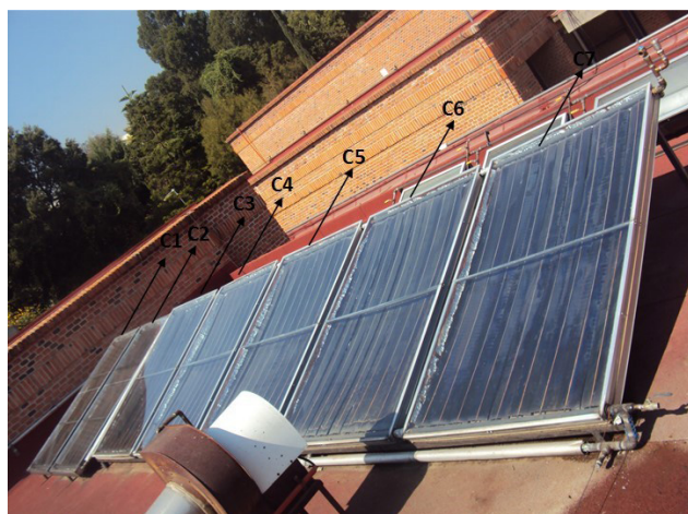
Fig. 2. Flat solar collector system.
