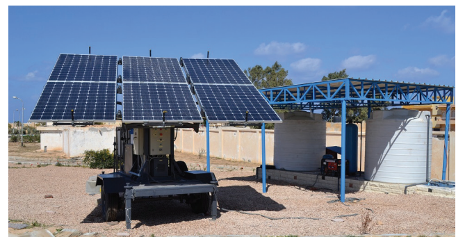
Fig. 2. Small mobile desalination system powered by renewable energy.
