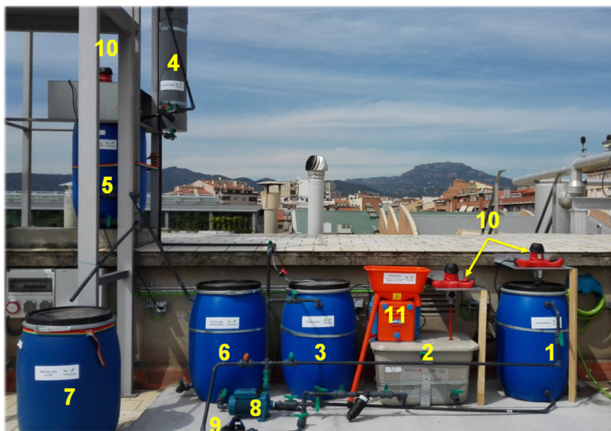
Fig. 2. Automated plant. 1) Water to treat container; 2) Coagulant preparation process; 3) Coagulant container; 4) Fast agitation; 5) Slow agitation; 6) Drinkable water; 7) Sludge; 8) Electric pump; 9) Manual pump; 10) Agitators; 11) Grinder.
