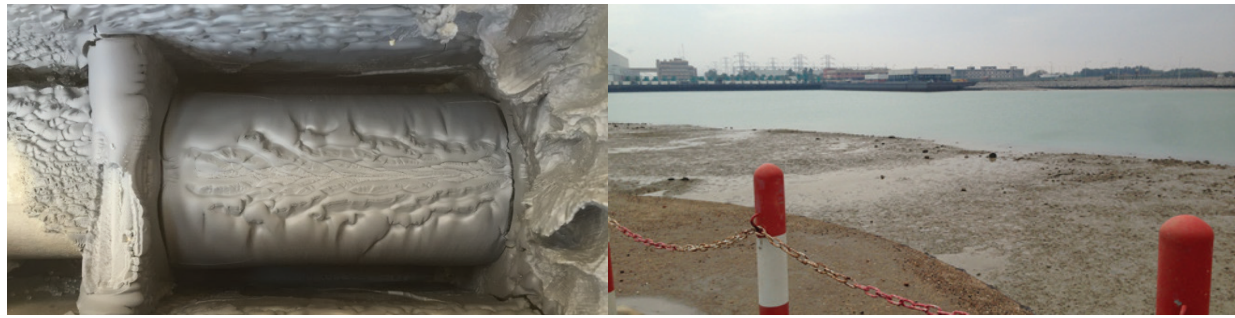
a.) heat exchanger covered with silt
