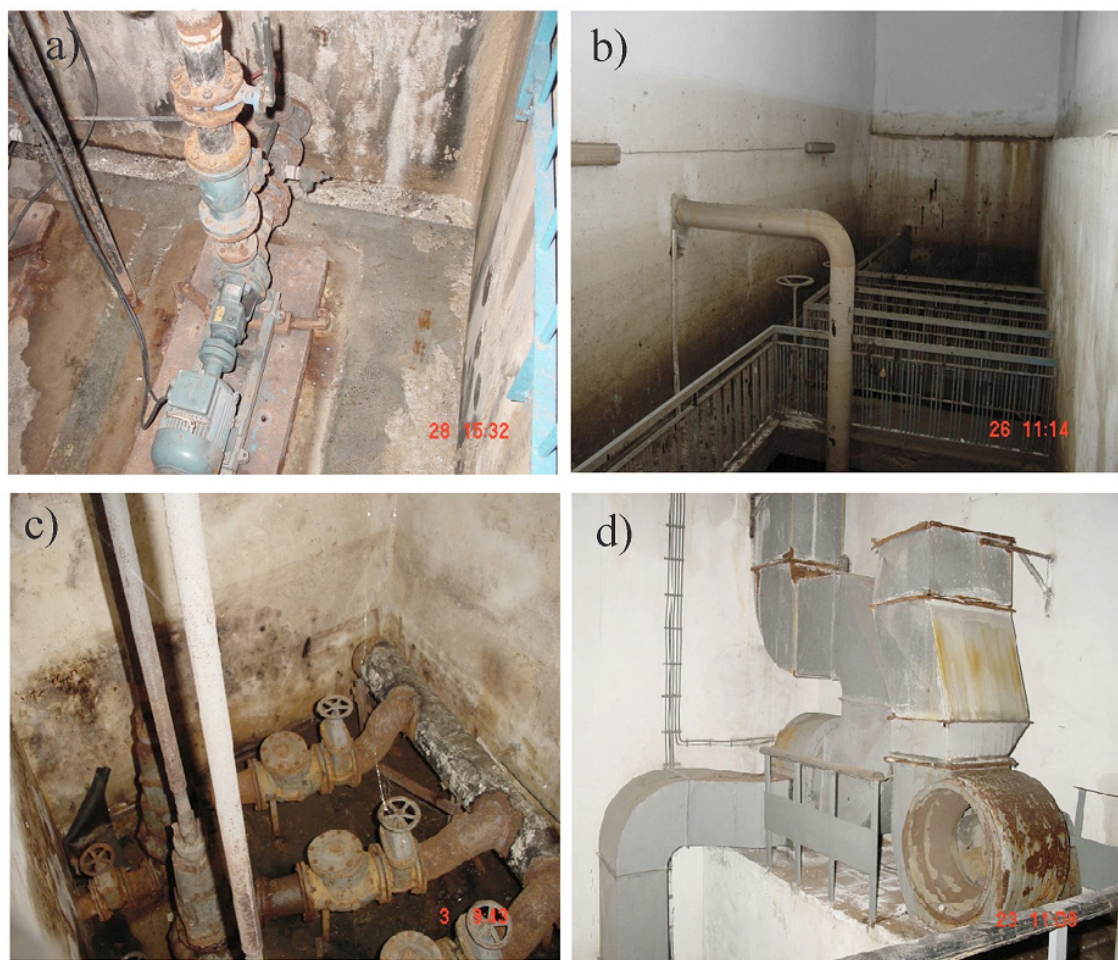
Fig. 4. (a) Concrete corrosion, (b) diver pumps, (c) concrete and steel corrosion and (d) ventilation with corrosion.
