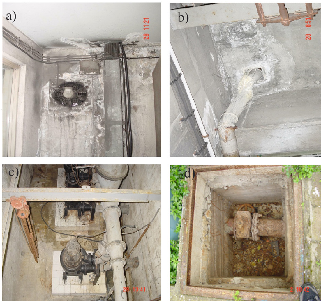
Fig. 3. (a) The damages of electric ports, (b) mechanical leakage of compression packing, (c) open screws and (d) armature bowl decayed.
