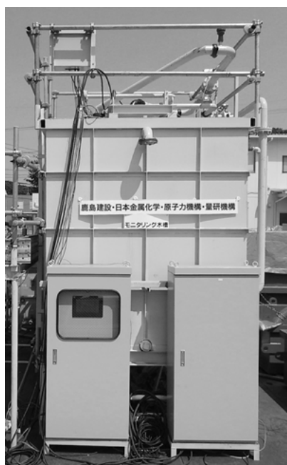
Fig. 1. Photo of the Cesimoni-water system.
