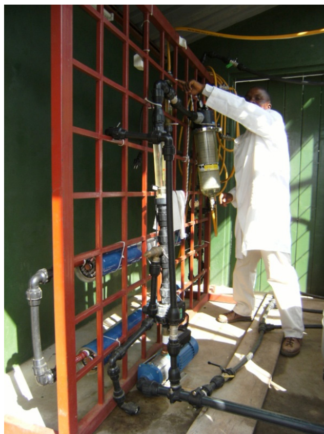
Fig. 6. UF plant installed at the Escola Primaria of Ressano García (Mozambique).
