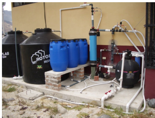
Fig. 2. UF plant set up in Girón (Ecuador).
