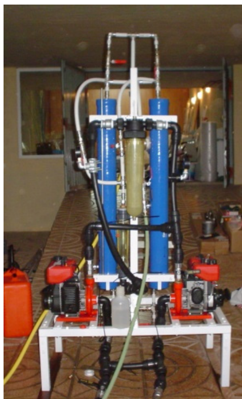
Fig. 1. UF plant set up in Pucará (Ecuador).
