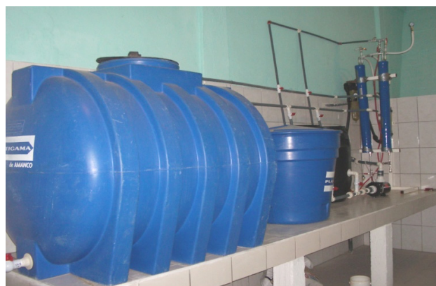
Fig. 3. UF plant set up in Santa Isabel (Ecuador).
