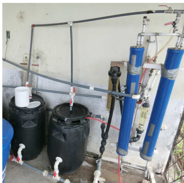
Fig. 4. UF plant set up in La Granja (Ecuador).
