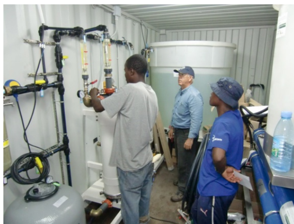
Fig. 7. UF plant installed at the Health Centre of Ressano García (Mozambique).
