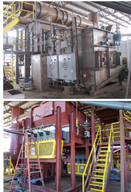
Fig. 4. Coaltec Energy gasification system at The Ohio Heifer Center.
