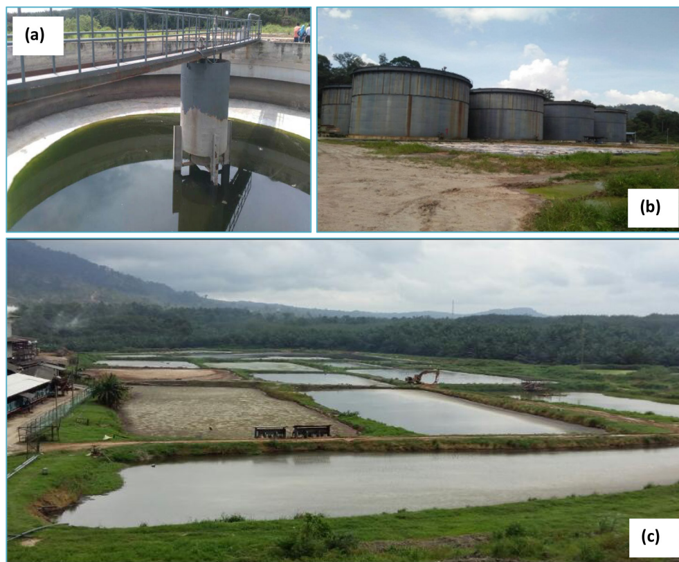
Fig. 3. (a) Mixing pond (b) Biogas tanks and (c) Ponding system.
