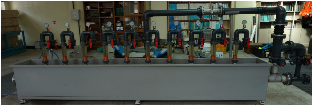
Fig. 3. Manifold pipe system for wet experiments.
