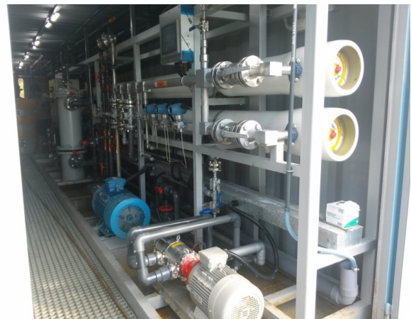
Actual installation in pilot plant
