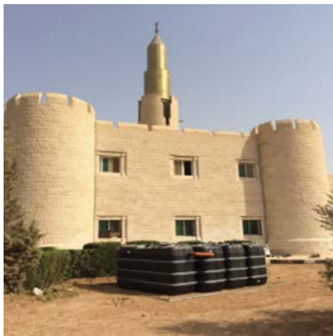
Fig. 2. Gray water treatment pilot plant at JUST Mosque.
