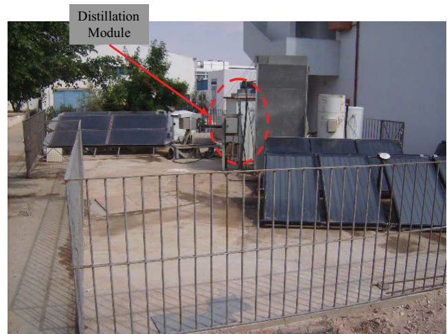
Fig. 11. A photo of the solar desalination unit experimental setup.
