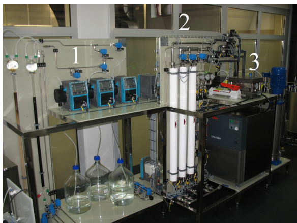
Fig. 1. (1) Ion-exchange system, nanofiltration modules with (2) spiral and (3) flat sheet membranes on the experimental stand in WWTP Janówek.
