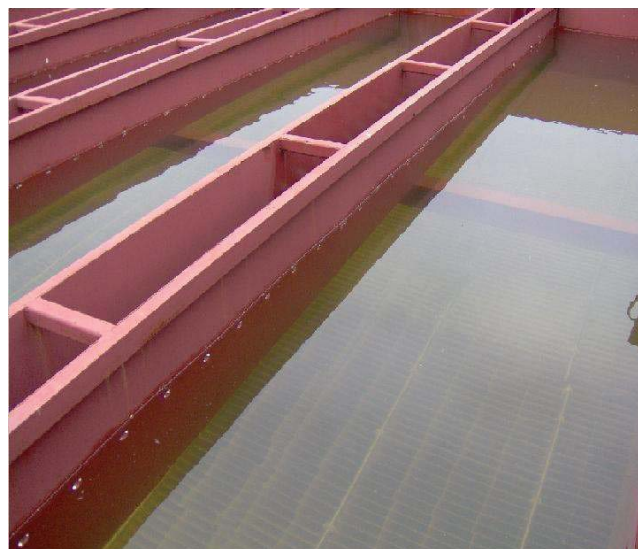
Fig. 10. Coagulating sedimentation tank.
