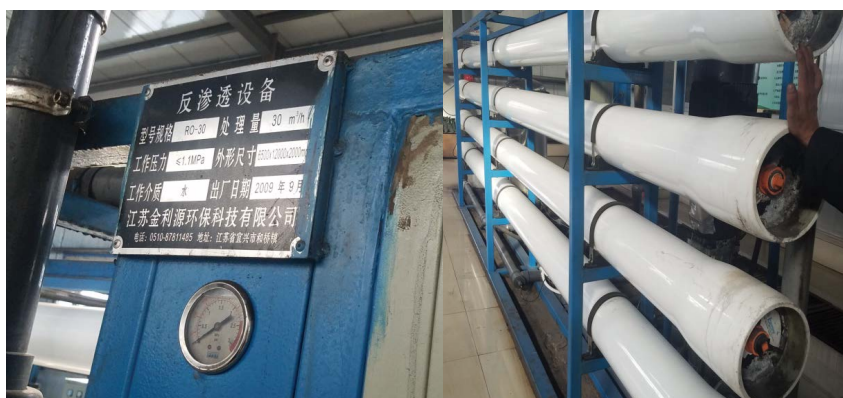
Fig. 16. Reverse osmosis system of mine water treatment in Wuhai City, Inner Mongolia.
