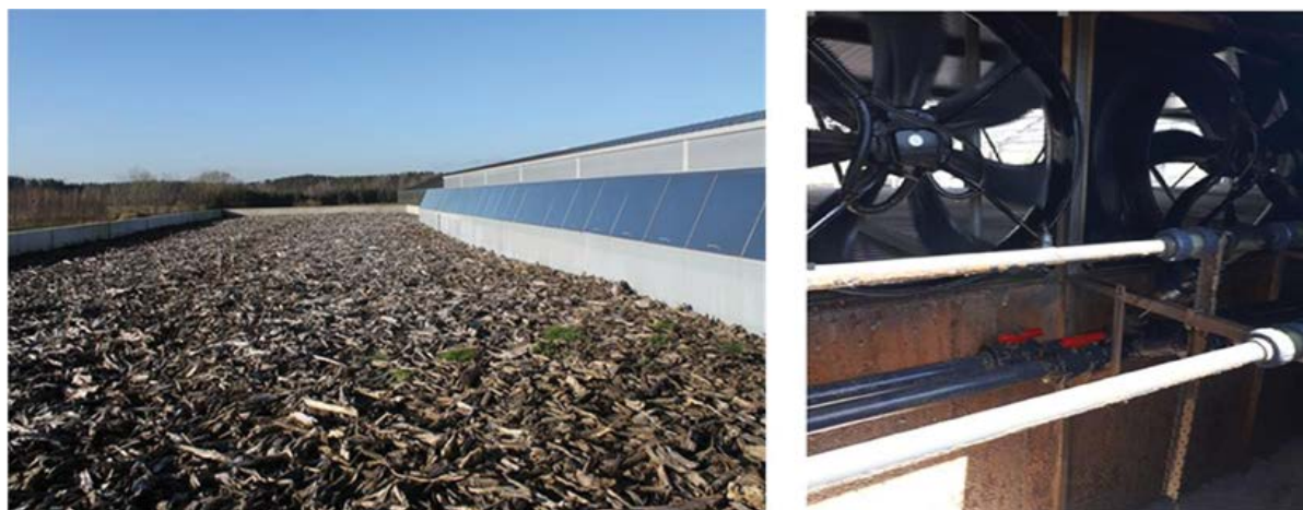
Fig. 3. View of the filling of the biofilter and the air supply channel from the dryer.
