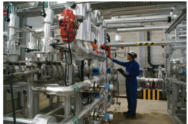
Fig. 2. 8" RO section of the testing asset.
