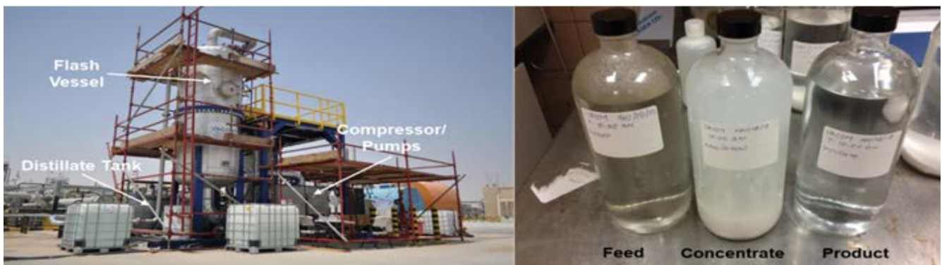
Fig. 12. Produced water desalination: mechanical vapour compression at field site.
