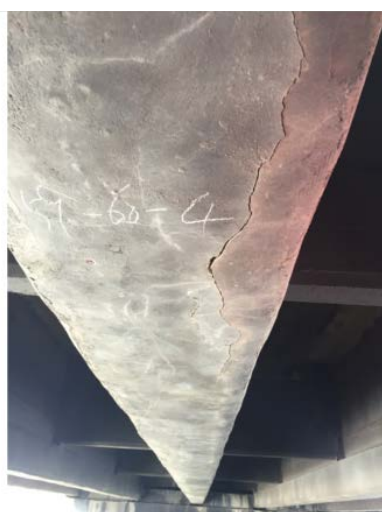
Fig. 3. Hollowing and cracking of T-beams.
