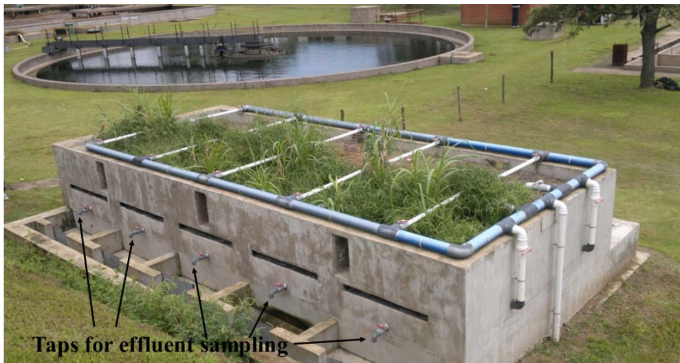
Fig. 4. Rhizofiltration unit at Kingsburgh showing about 80% plant cover on the planted section, 3 months after the initial planting of the macrophytes. Arrow indicates the sampling points.
